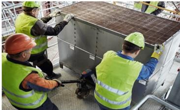
Installation stationary DNOx catalyst
